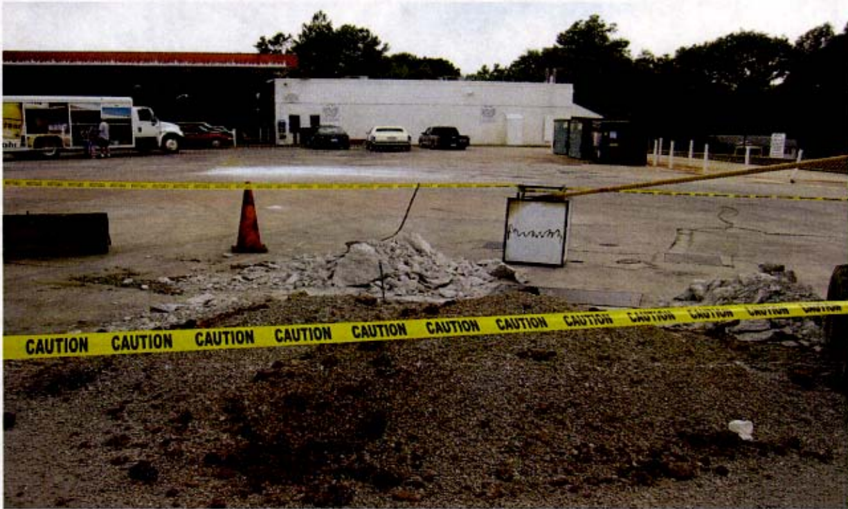
Photo 3. View of excavated soil and gravel north of diesel fuel dispenser island.
