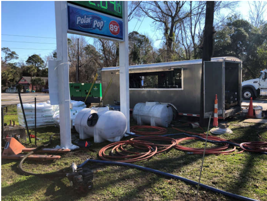
Photo 6: Magnesium sulfate and magnesium sulfate solution tank, fresh water tank and mixing/injection system 2/24/21
