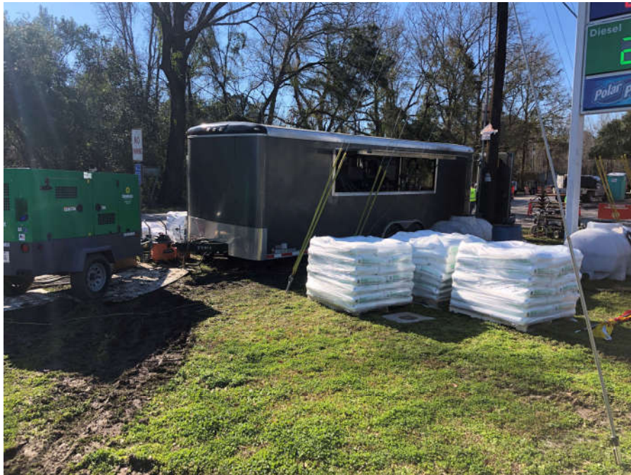
Photo 4: Injection system and equipment staging 2/24/21
