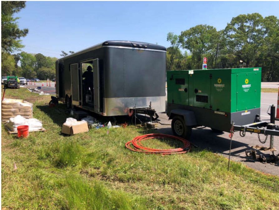
Photo 16: Injection equipment and materials set up for injection on southbound shoulder of US-17 4/7/21
