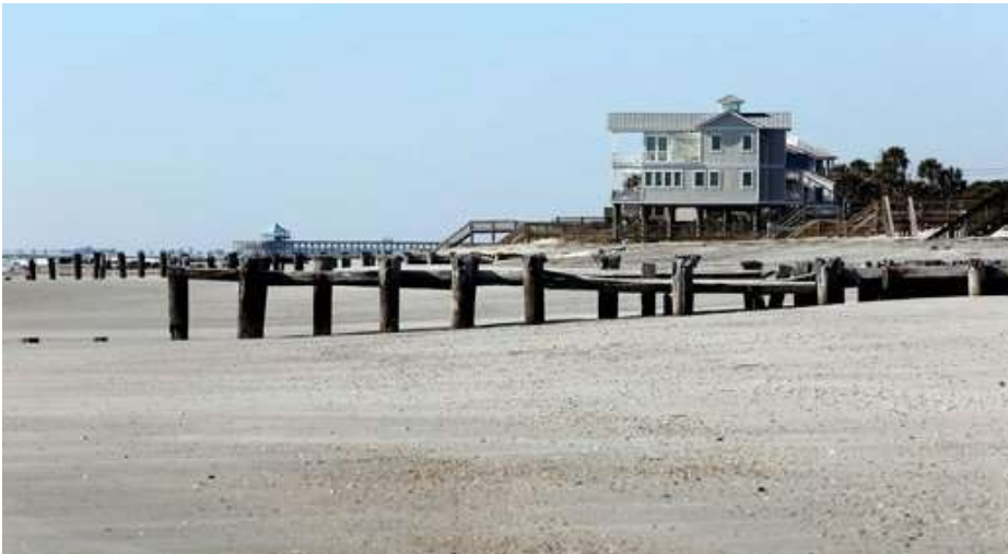
FIGURE 37. PHOTO OF A DILAPIDATED TIMBER-PILE GROIN ON FOLLY BEACH.
