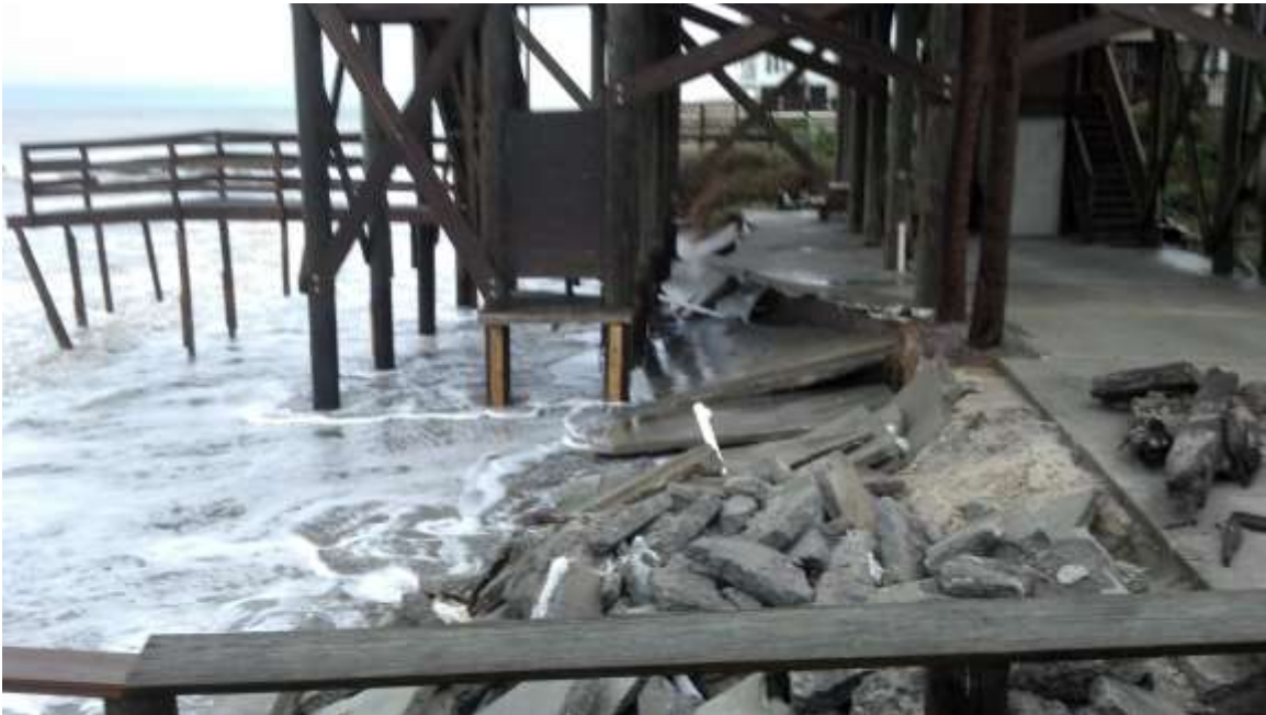
FIGURE 41. PROPERTY DAMAGE ON THE NORTHEAST PORTION OF FOLLY BEACH DUE TO EROSION CAUSED BY HURRICANE SANDY IN 2012.
