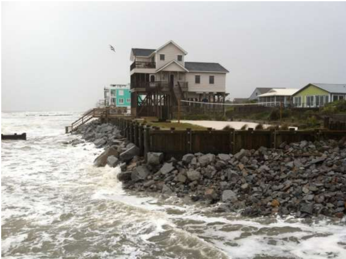
FIGURE 26. EXPOSED SEAWALL AT SUMTER AVE. ALONG THE NORTHEASTERN PORTION OF FOLLY BEACH PRIOR TO THE FEDERAL RENOURISHMENT PROJECT IN 2014.
