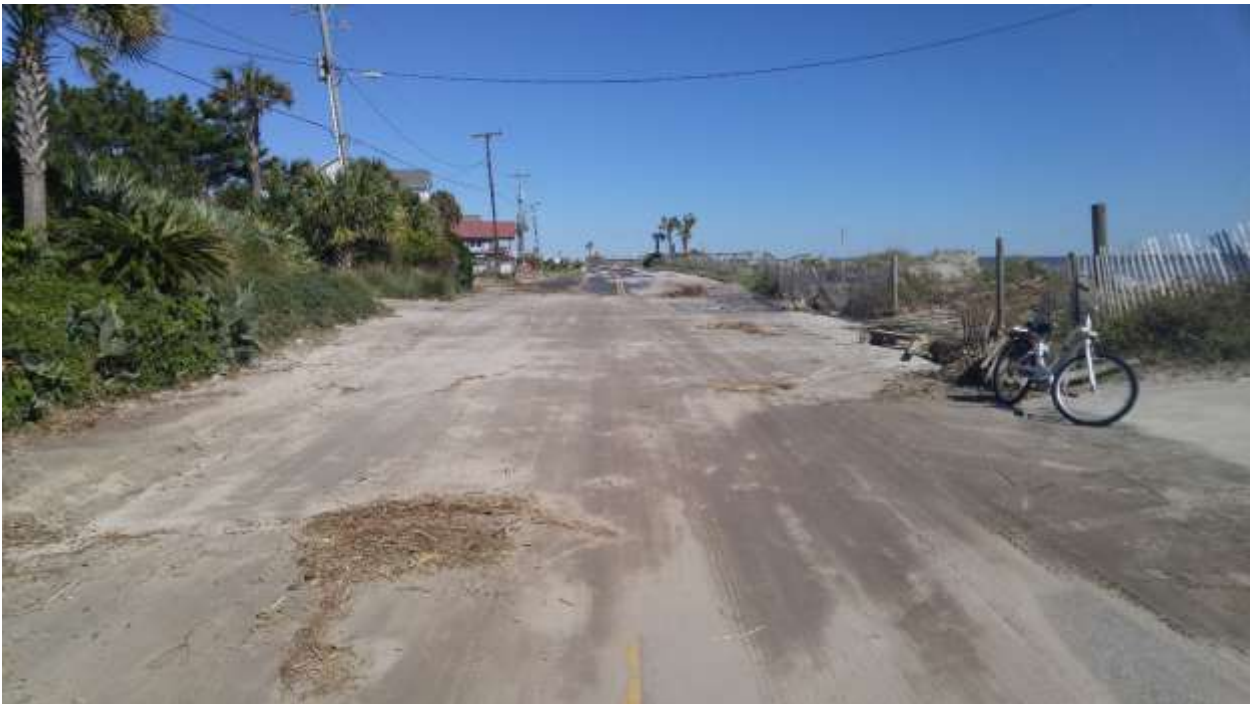
FIGURE 42. FOUR PHOTOGRAPHS OF THE POST-MATTHEW CONDITION OF THE BEACH AND EAST ASHLEY DR AT THE WASHOUT, TAKEN ON OCT 9, 2016.
