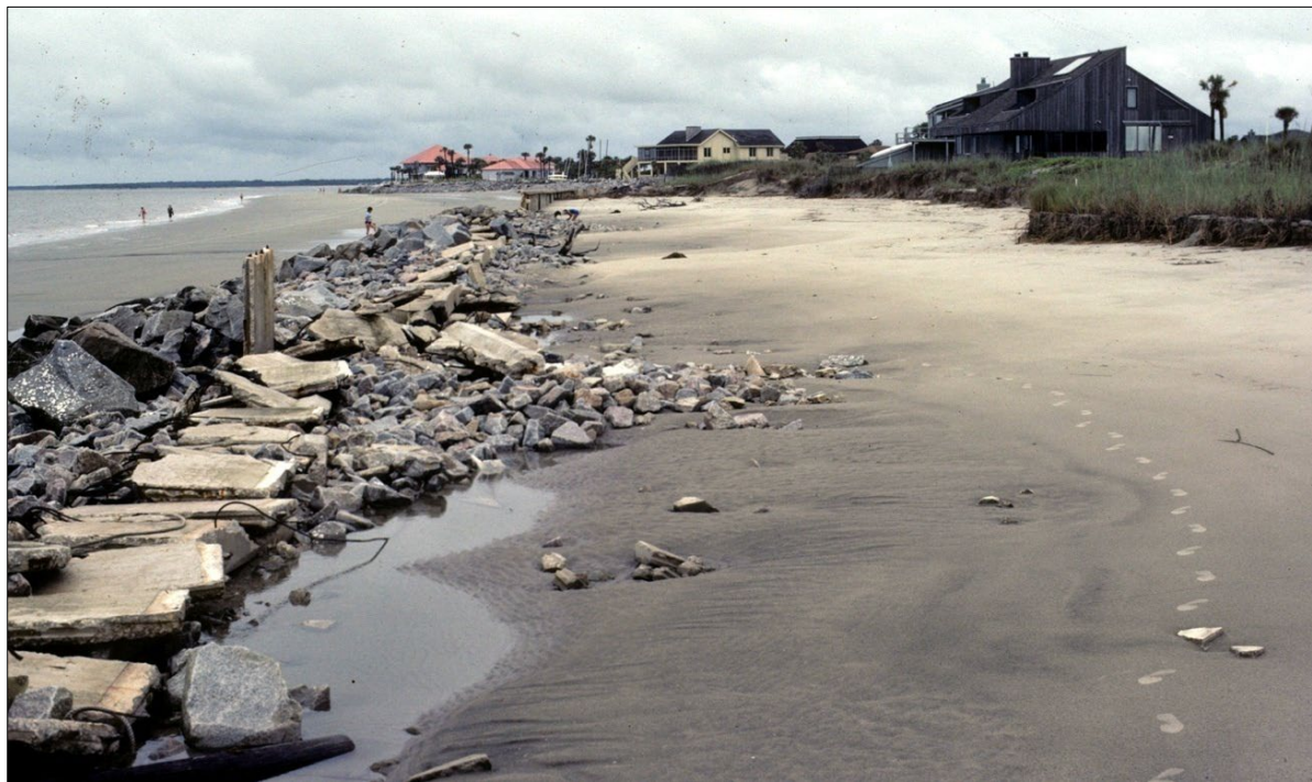
FIGURE T-8. Encroachment (upper) of the northern channel (deep blue area) of North Edisto Inlet and lack of maintenance led to collapse (lower) of a section of seawall near Beach Court in 1983.
