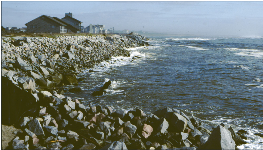
FIGURE 3.6. Beach erosion along North Beach led to exposed seawalls, no recreational beach, and severe damage to structures in 1983. View north along Renken Point in 1985 at low tide. [After CSE 1989]
