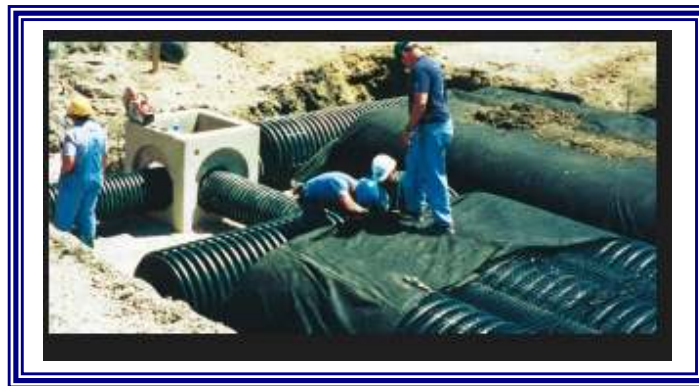
HDPE Underground Detention
