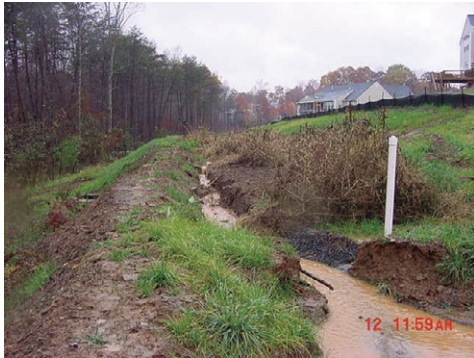
Bioretention swale, installed too early during active construction, has become clogged with sediment.
