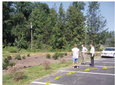
Some site runoff by-passes bioretention because of inadequate slope of filter strip.
