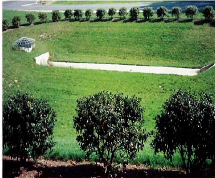
Figure 4-2: Detention (Dry) Pond
