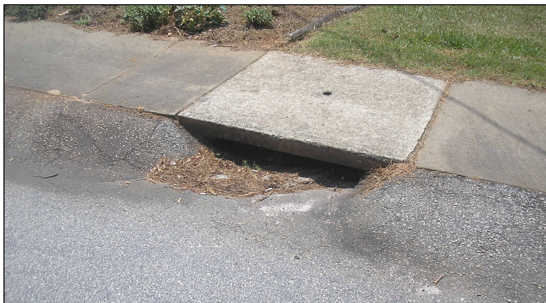
Fig. 25. Catch basin with landscape and natural debris in the basin.
