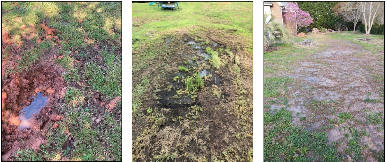
Failing septic drain fields in the 3&20 Creek (left) and Tyger River (center and right) watersheds.
