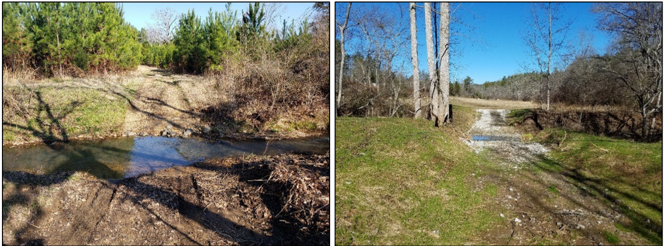
Examples of stabilized ford crossings: dirt road (left), crushed gravel (right). Source: SCFC.
