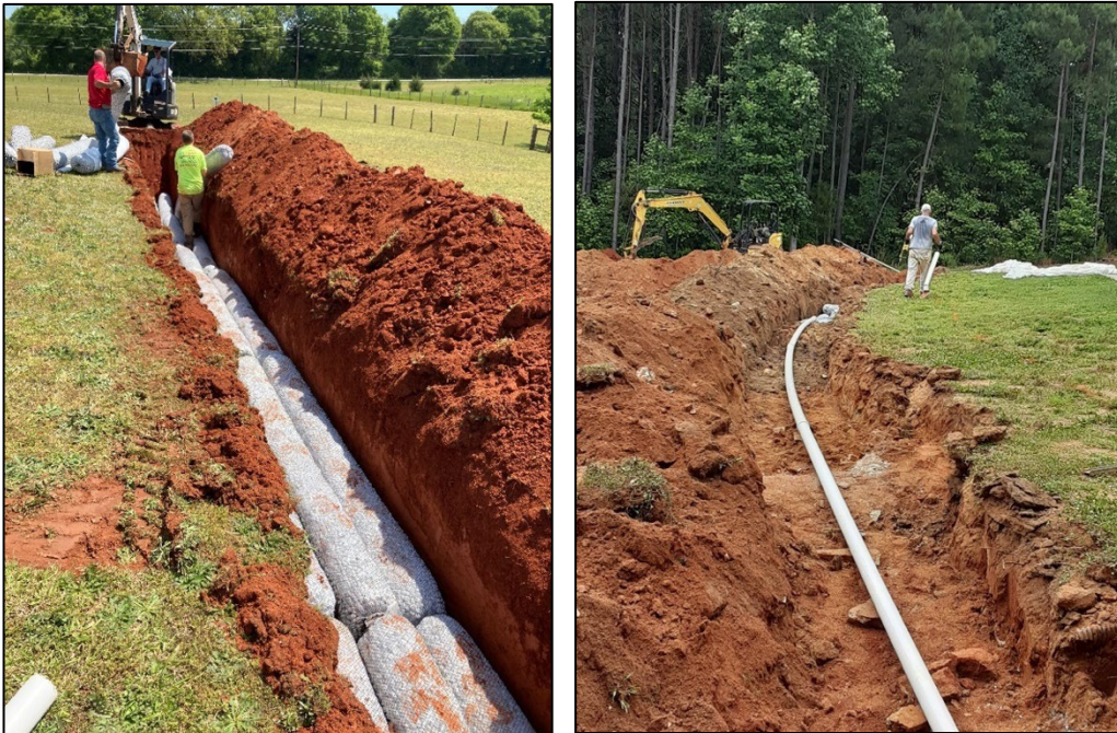
Examples of septic drain-line repairs in the 3&20 Creek Watershed. EZ-flow pipe (left), outlet pipe (right).
